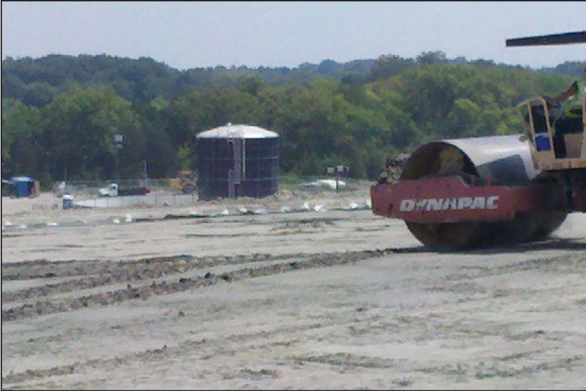
6K - Roller compaction of ash material in lifts at the Arrowhead Landfill, Uniontown, AL. August 26, 2010.
