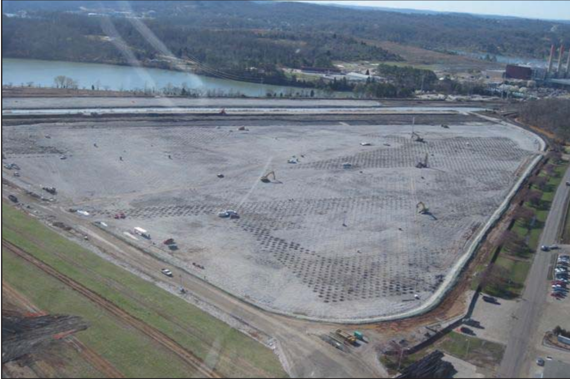
3A - Ball Field construction during installation of wick drains on grid pattern. March 20, 2009.
