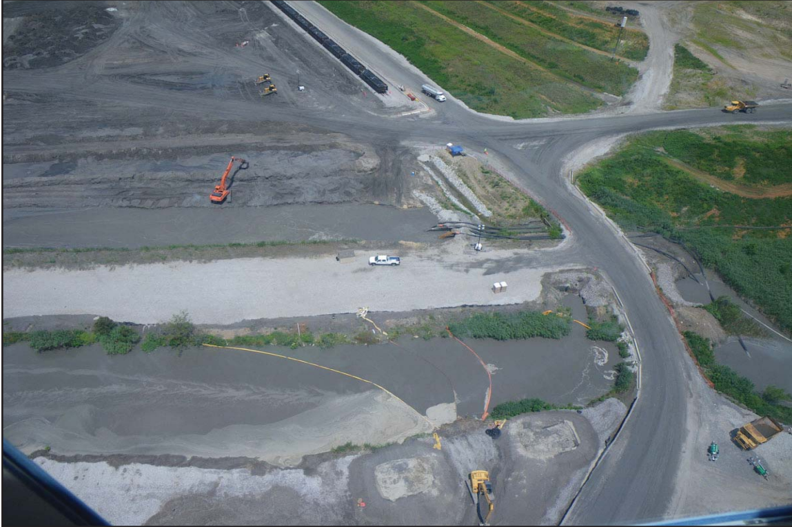
3C - Dredged ash processing showing discharge to Rim Ditch (top) and from Sliuce Trench (bottom). July 1, 2009.
