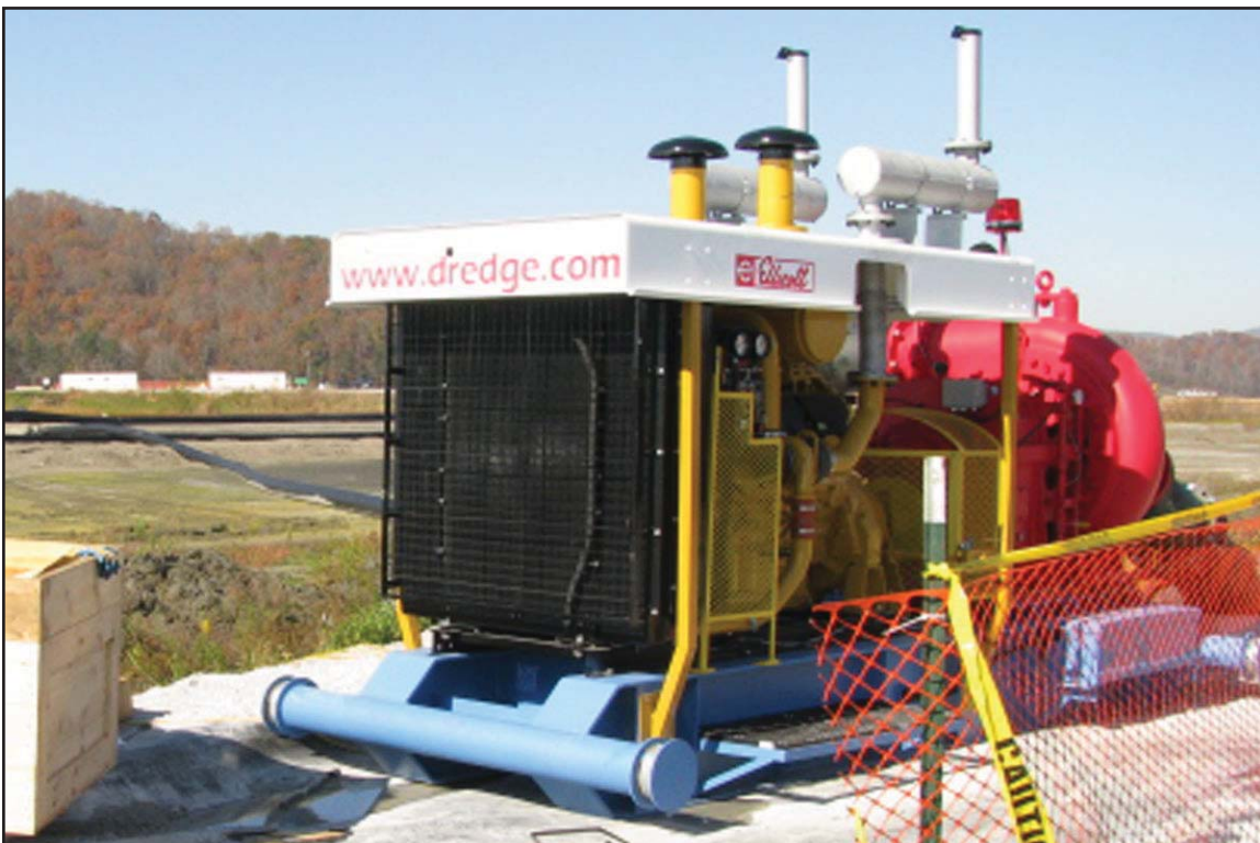
2P - Dredge discharge line booster pump showing noise muffler. November 7, 2009.
