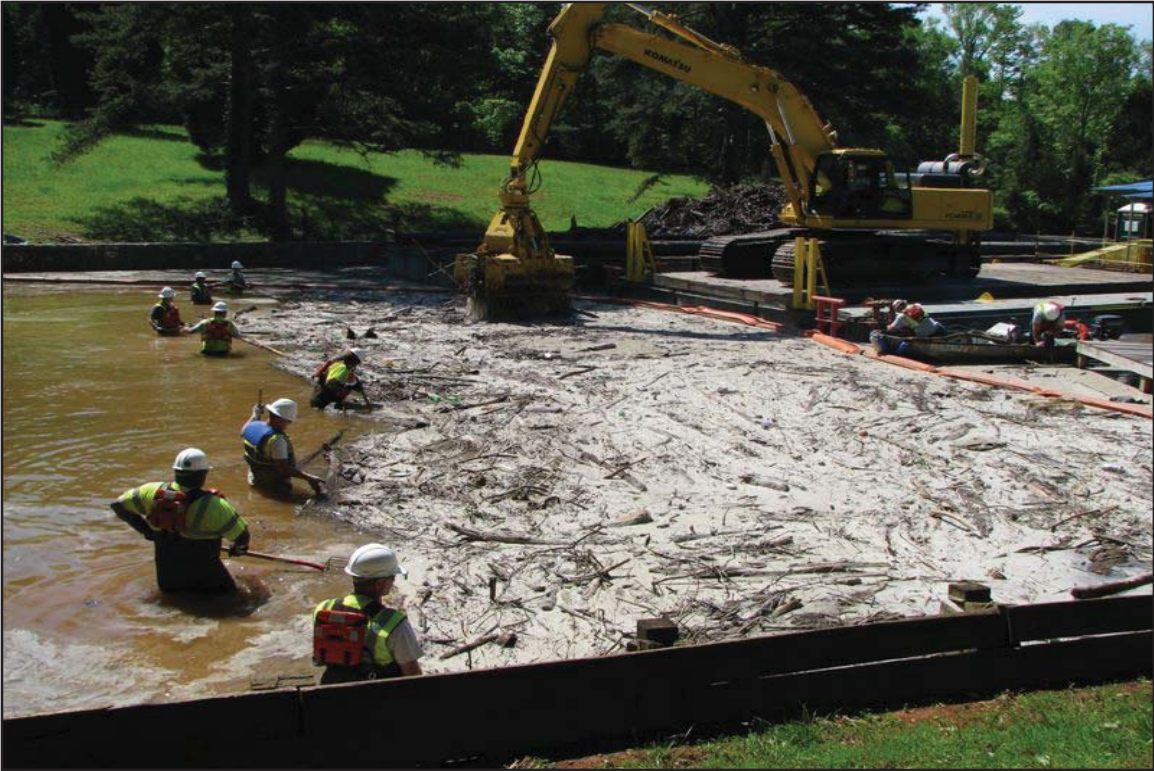
7C - Workers and mechanical excavators used to remove trapped cenospheres and debris from cove. May 11, 2009.
