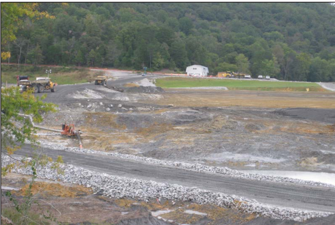
4H - Excavation east of Dike 2 nearing bottom of excavation (Dike 2 at left). October 6, 2009.
