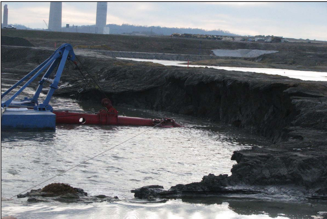
4N - Removal of ash dike separating Swan Pond Embayment from Emory River. January 14, 2010.
