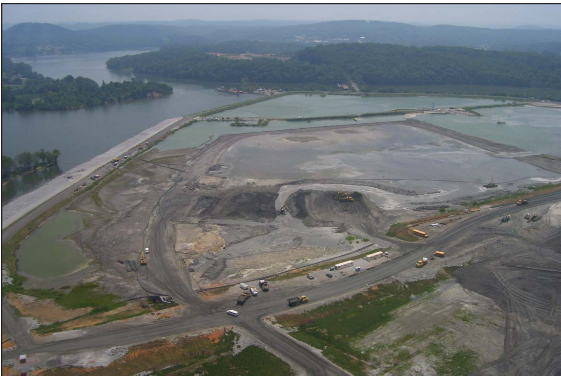
3N - Lateral Expansion Area converted to use for wet ash storage and ash recovery from Ash Pond dredge discharge. July 8, 2010.
