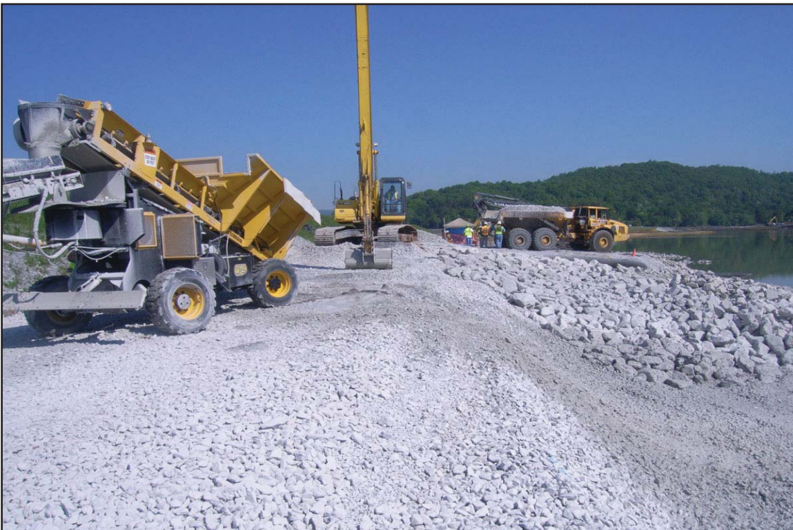
8H - Equipment used in placing sand, gravel, and riprap during Dike C reinforcement. April 29, 2010.
