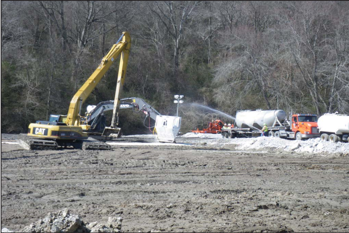
4O - Addition of lime during excavation of East Embayment to reduce moisture content in the ash. March 4, 2010.
