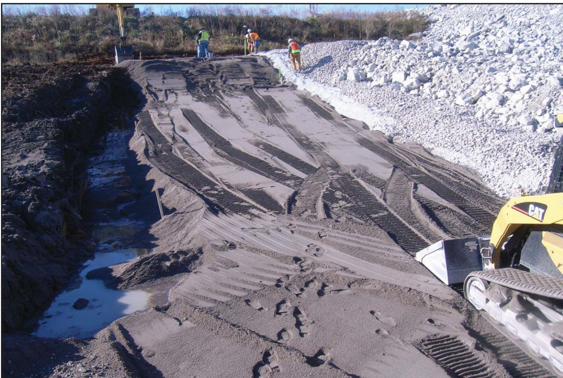
8B - Placing layer of sand on top of dike material in panel. December 29, 2009.
