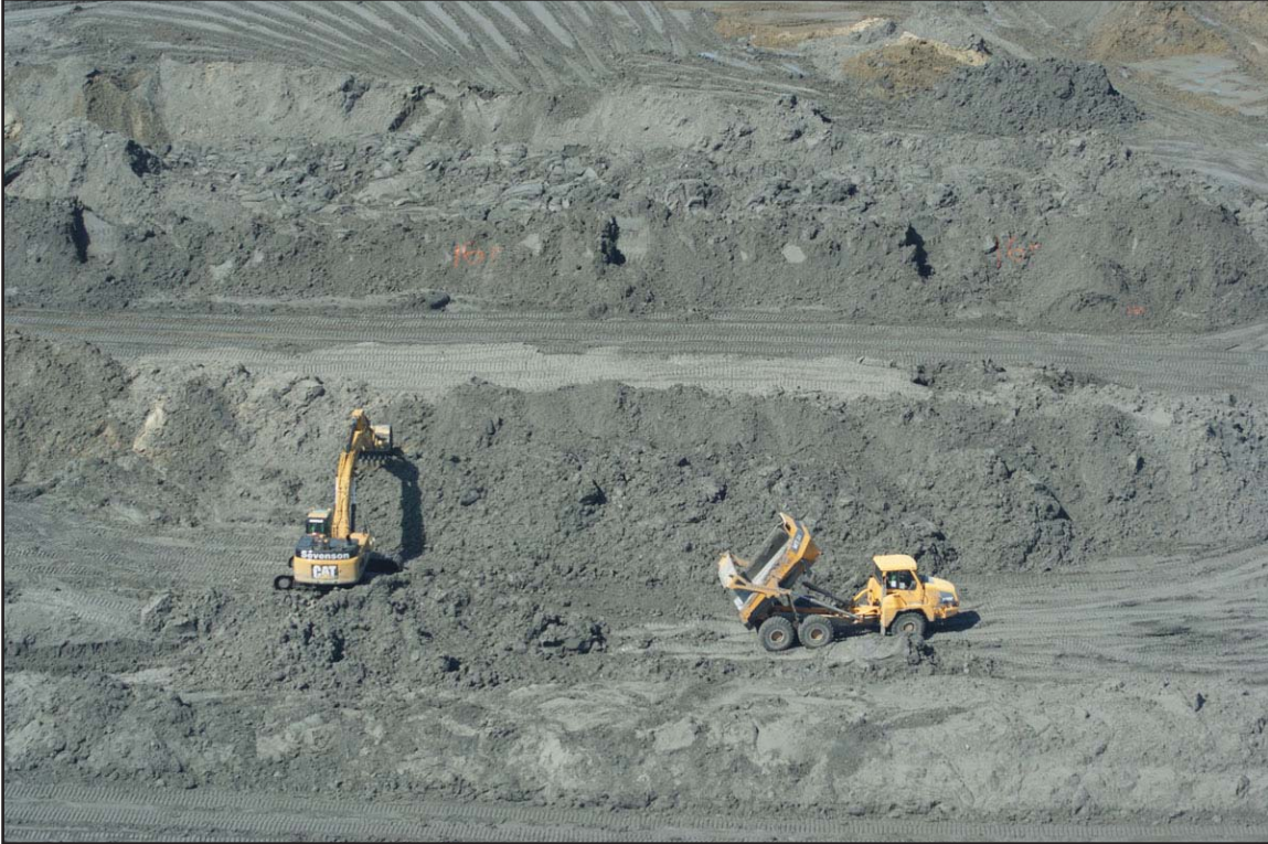
3G - Equipment in the Ball Field continuously moving ash in windrows to aid in drying. October 8, 2010.
