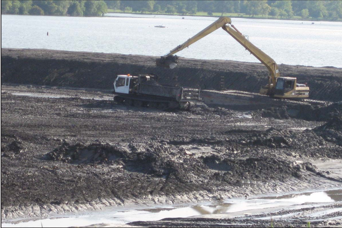
4C - Amphibious long-neck backhoe excavator and tracked dump truck used to excavate ash east of Dike 2. August 31, 2009.
