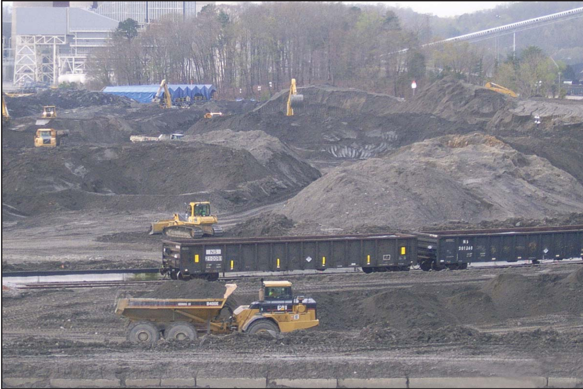
3I - Equipment in the Ball Field continuously moving ash in windwors to aid in drying. April 5, 2010.
