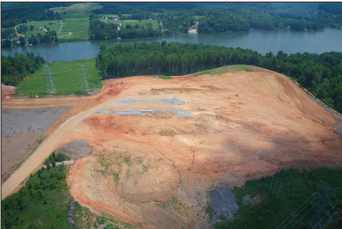
5D - Peninsula Storage area, constructed as alternate temporary storage site, but never used. July 2, 2009.
