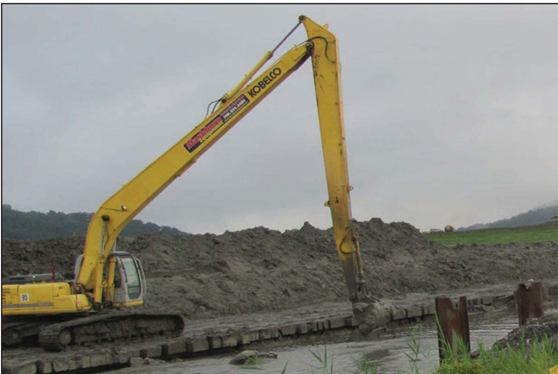
3D - Dipping (excavating) dredged ash from Rim Ditch, showing sheet pile wall. April 10, 2010.
