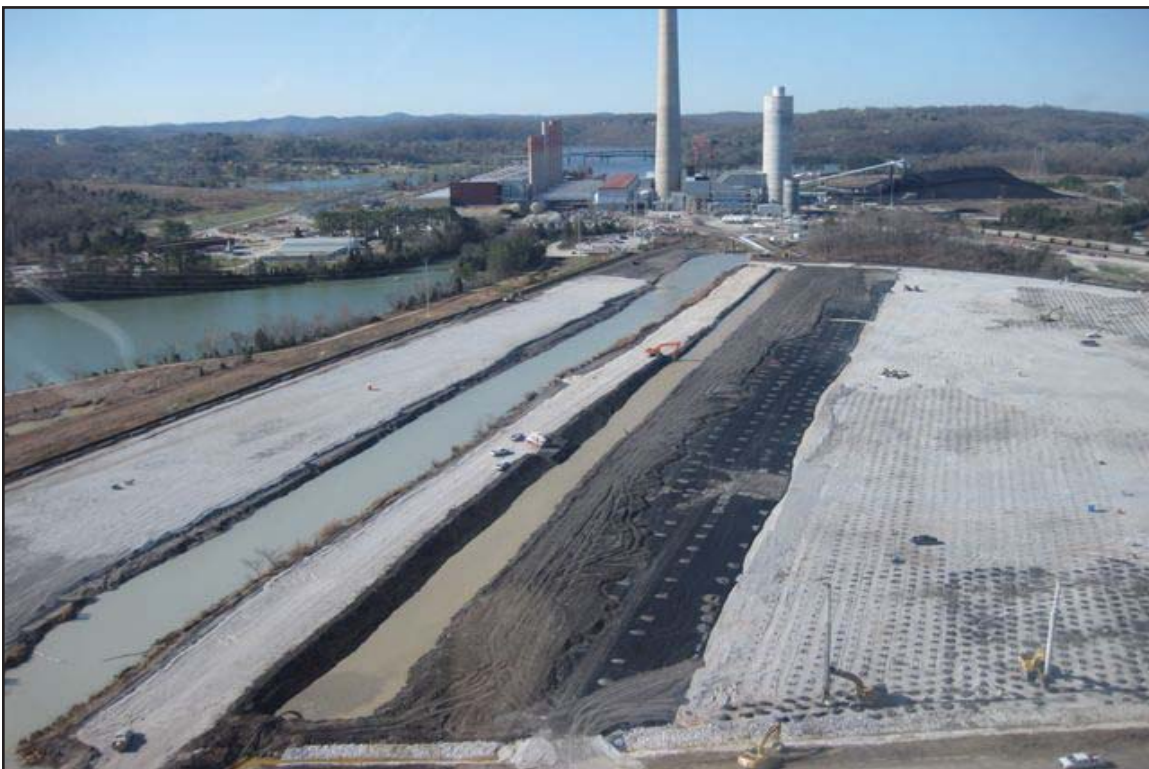
3B - Ball Field construction during installation of wick drains and gravel demarcation layer. March 30, 2009.
