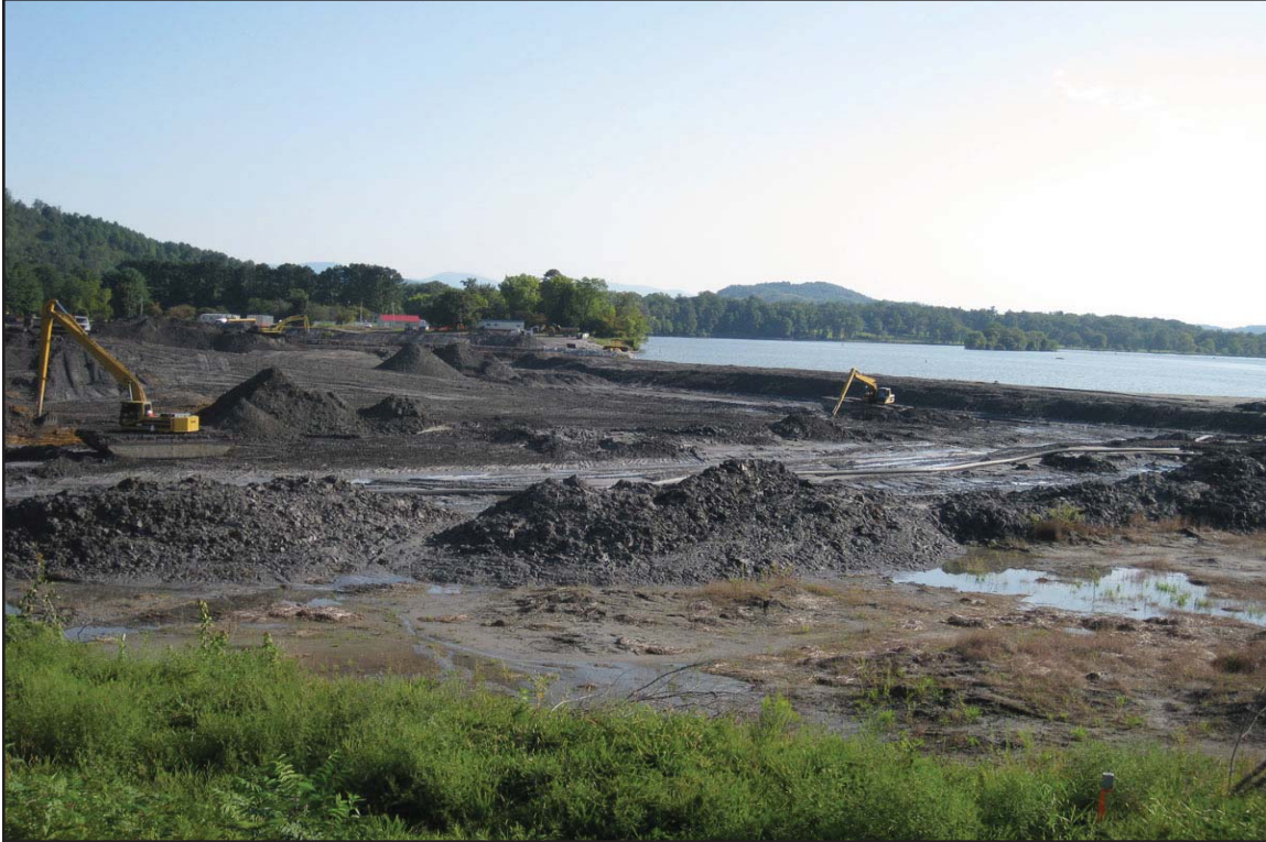
4A - Excavation east of Dike 2 showing ash dike separating work area from Emory River. August 31, 2009.
