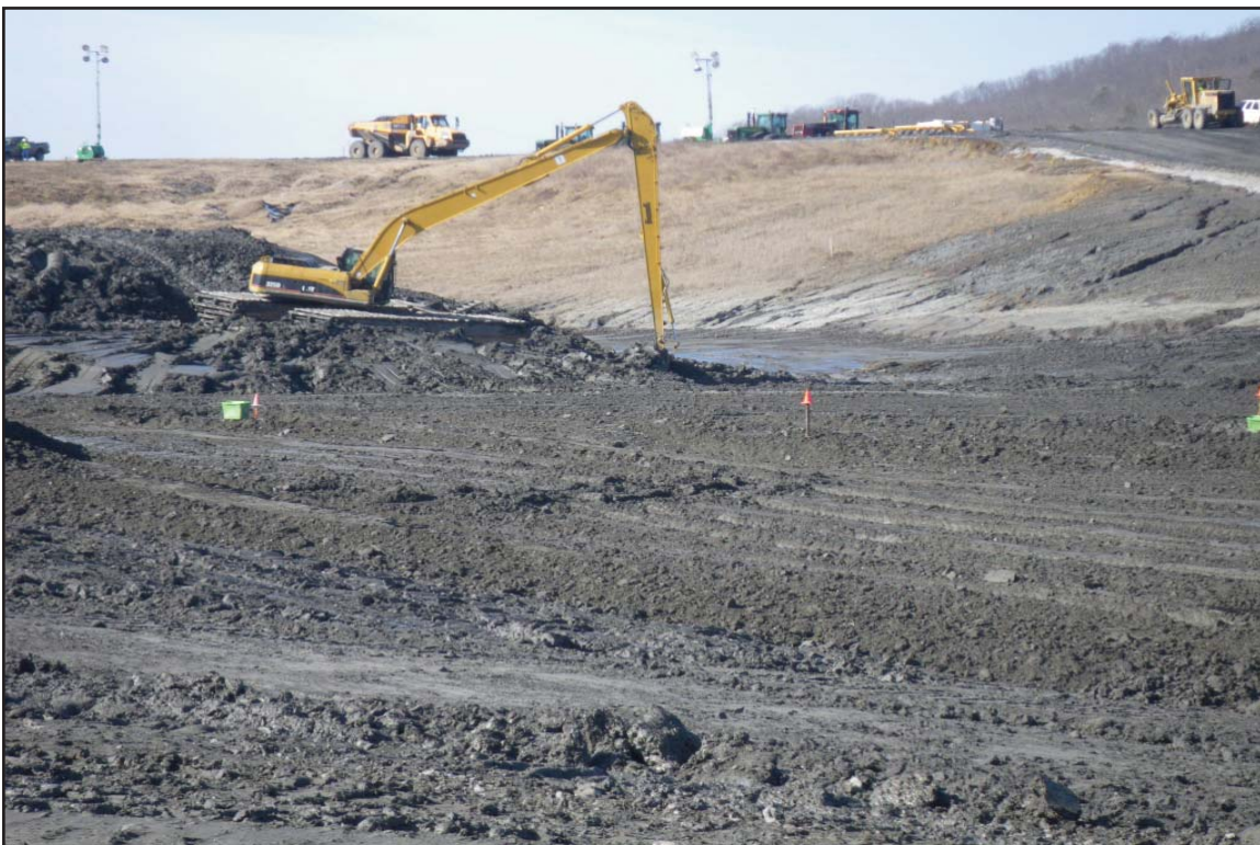
5F - Temporary storage of wetter ash in "valley area" of Dredge Cell next to Dike D. February 19, 2010.
