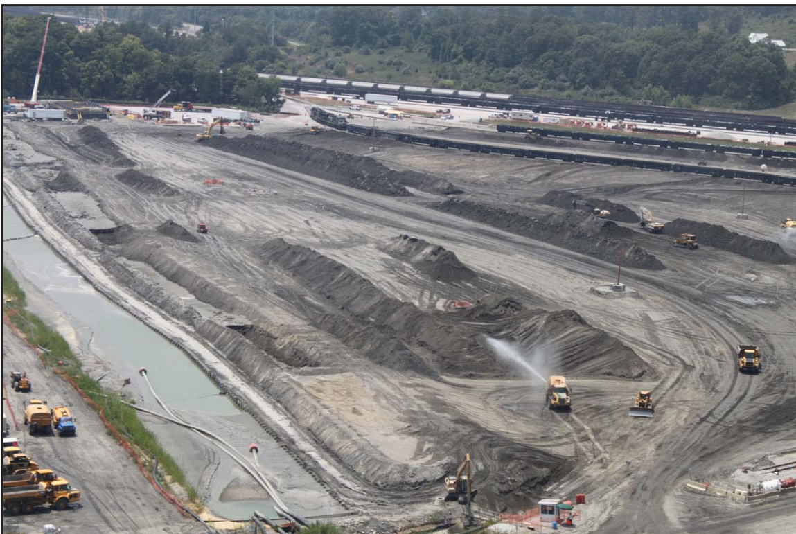
3F - Dewatering ash in the Ball Field using windrows (piles of ash in long rows). July 8, 2010.
