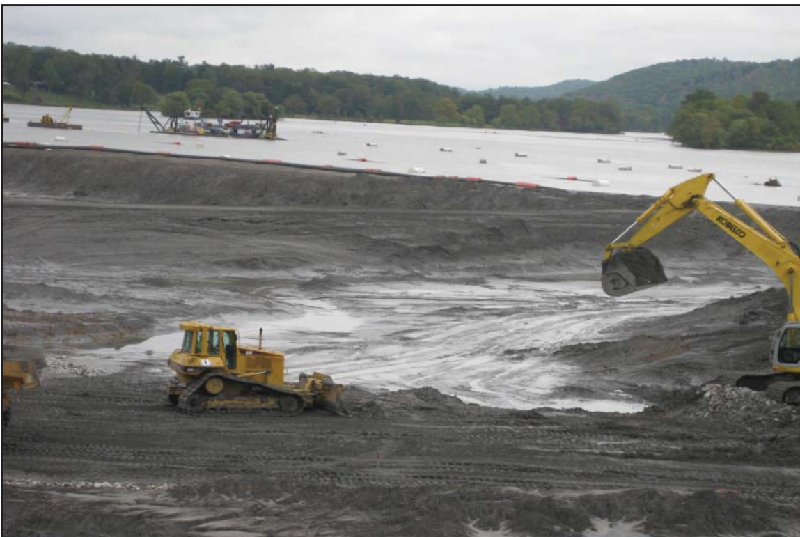
4F - Excavation east of Dike 2 nearing bottom of excavation in Swan Pond Embayment. October 6, 2009.
