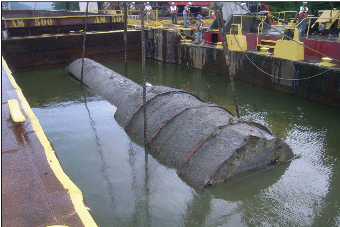
7J - Removal of skimmer wall debris at the Kingston Fossil Plant intake channel. June 5, 2010.
