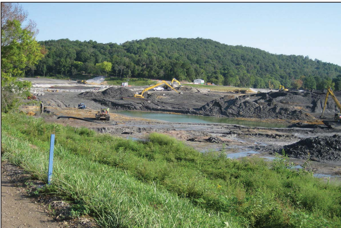
4B - Excavation east of Dike 2 showing riprap-lined Dike 2 haul road (left). August 21, 2009.
