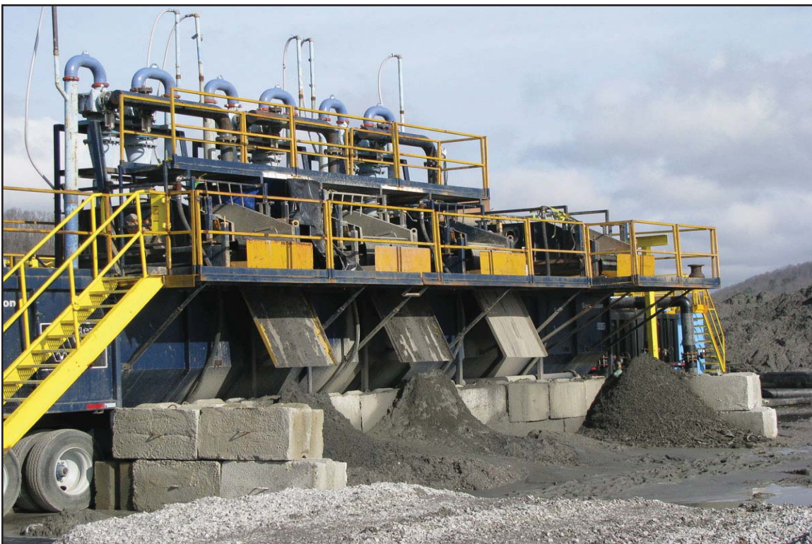
3P - Filter presses used for ash recovery from Ash Pond dredge discharge. January 23, 2010.
