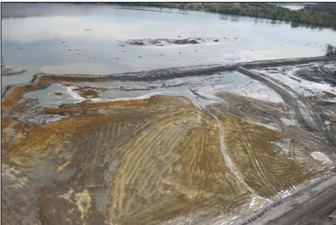
4J - Excavation east of Dike 2 nearing bottom of excavation (ash dike separating from Emory River at top). October 9, 2009.
