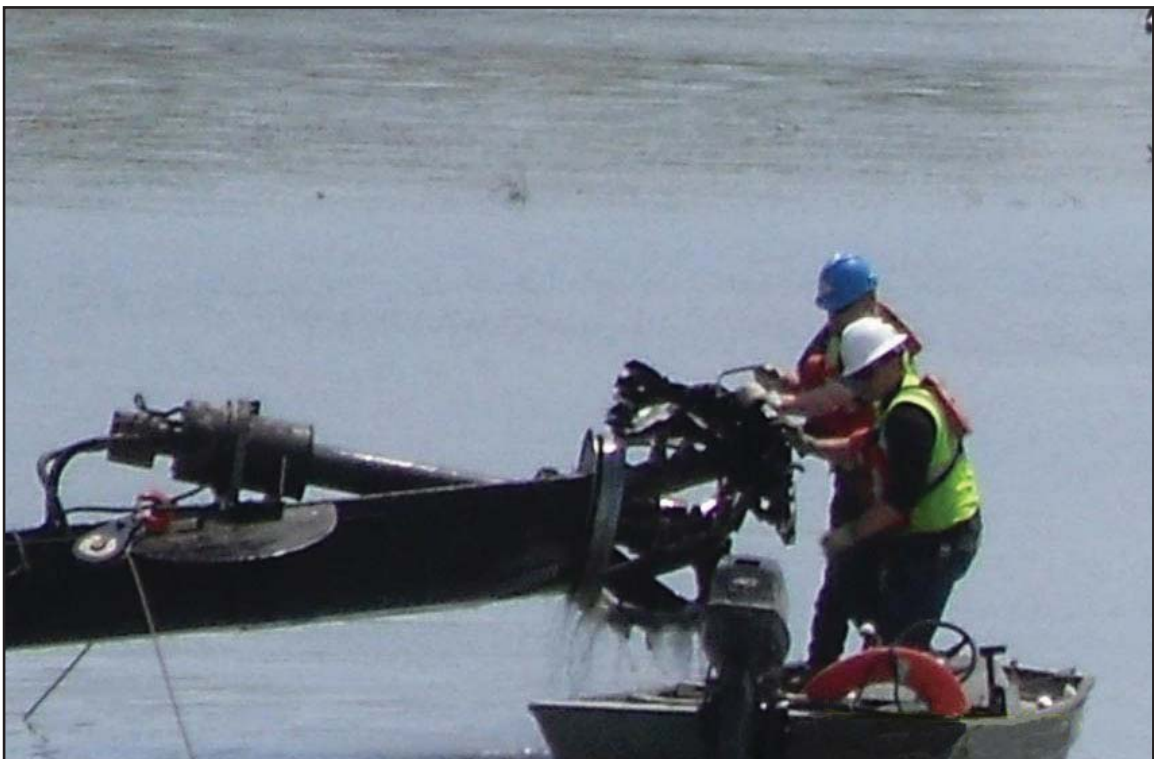
2B - TransAsh Emory dredge cutter head; Southern Shores workers removing debris. April 24, 2009.
