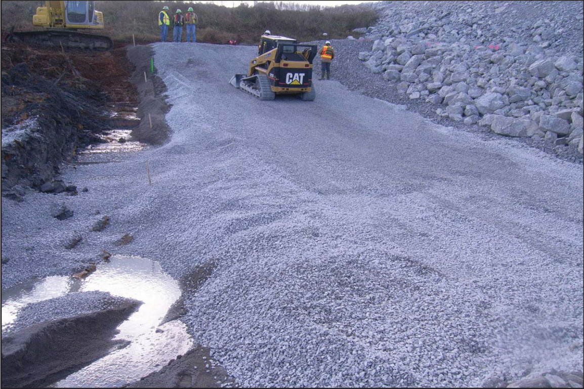
8C - Placing layer of gravel on top of sand material in panel. December 27, 2009.
