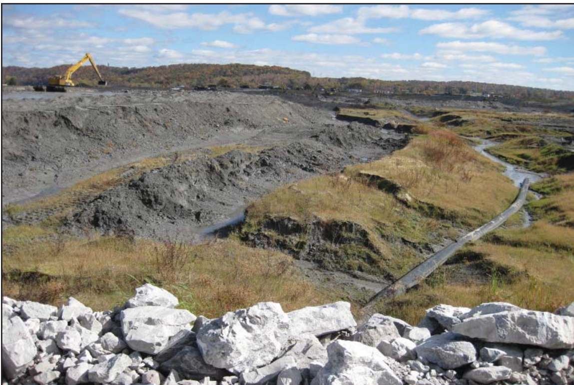
5B - West Storage Area, temporary dry ash storage for materials excavated east of Dike 2. October 28, 2009.
