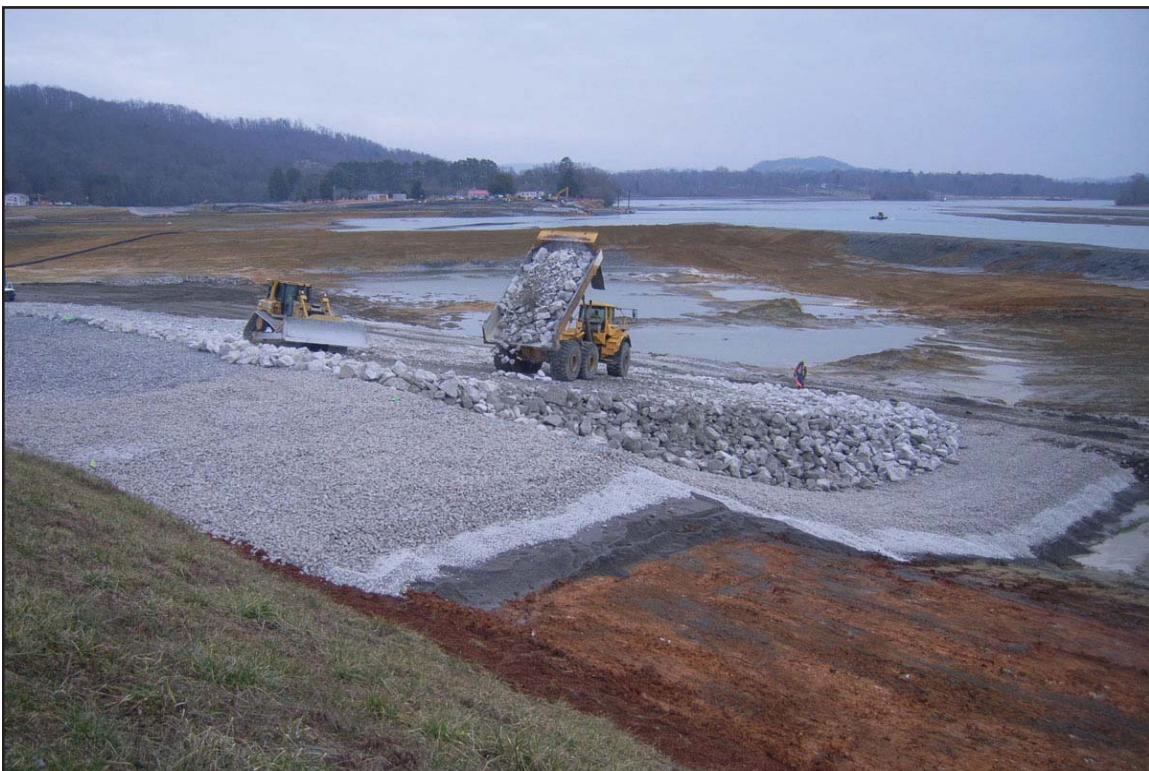
8F - Progress of overall Dike C reinforcement work as viewed from top of Dike C. February 24, 2010.
