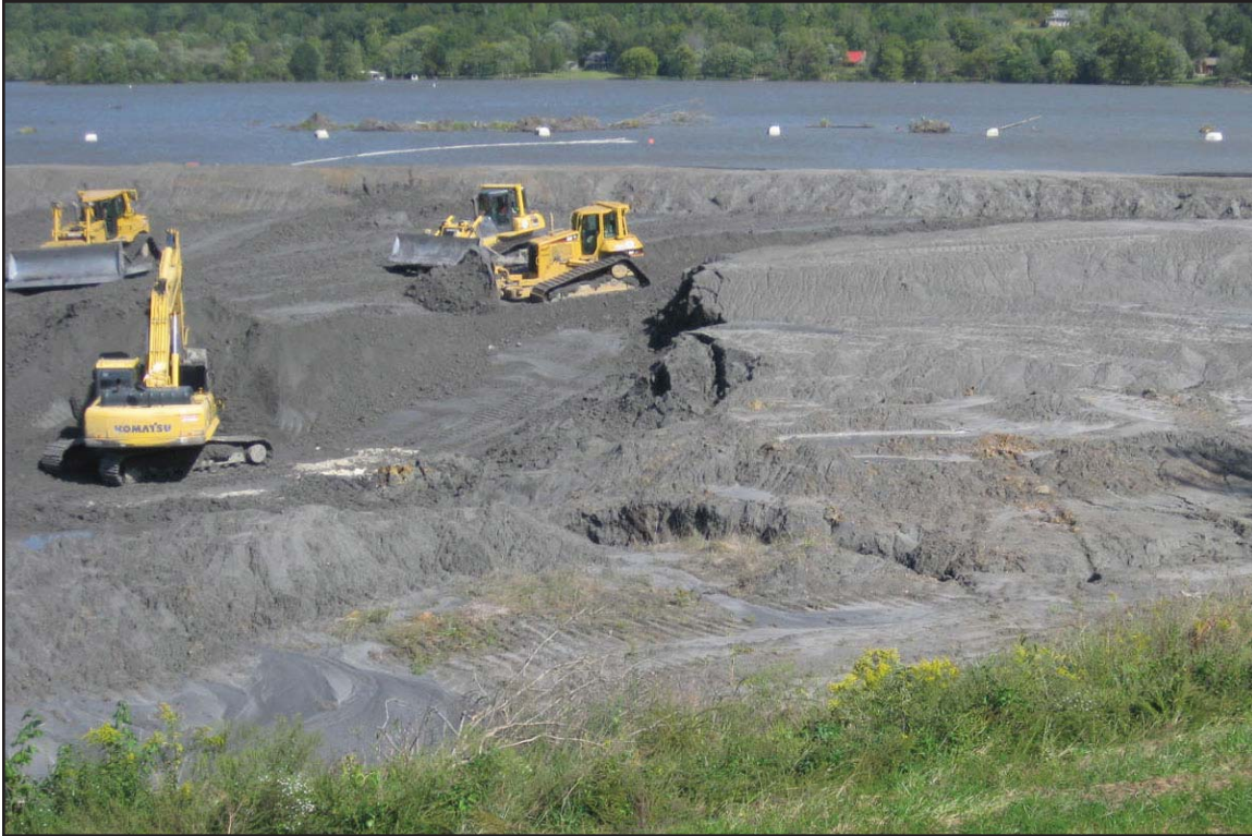
4E - Excavation east of Dike 2 using track-mounted bulldozers and backhoe excavators. September 28, 2009.
