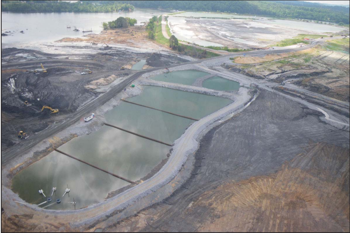
10C - Sediment basins used to settle out ash particles from dirty water ditch stormwater flows. July 2, 2009.
