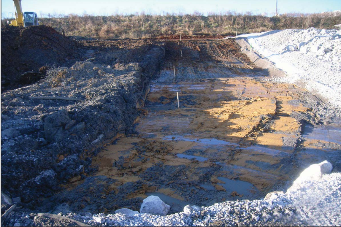
8A - Excavating ash in “panels” from outboard slope of Dike C to expose dike material. June 5, 2010.
