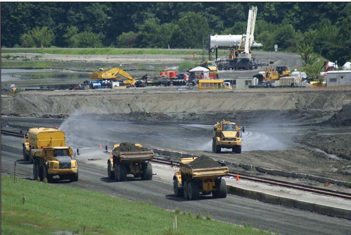
10H - Water spraying to control dust on haul roads and exposed ash surfaces. July 13, 2010.
