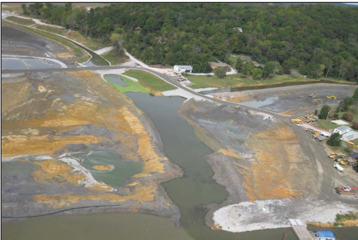
4L - Excavation east of Dike 2 nearing bottom of excavation (East Embayment at right). October 9, 2009.
