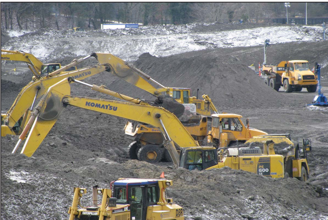
3H - Equipment in the Ball Field continuously moving ash in windrows to aid in drying. January 8, 2010.
