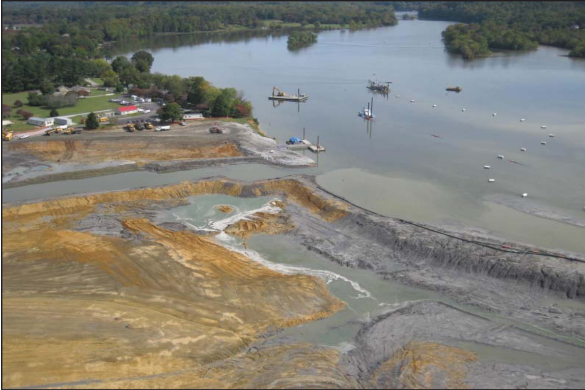
4K - Excavation east of Dike 2 nearing bottom of excavation (ash dike separating from Emory River at top). October 9, 2009.
