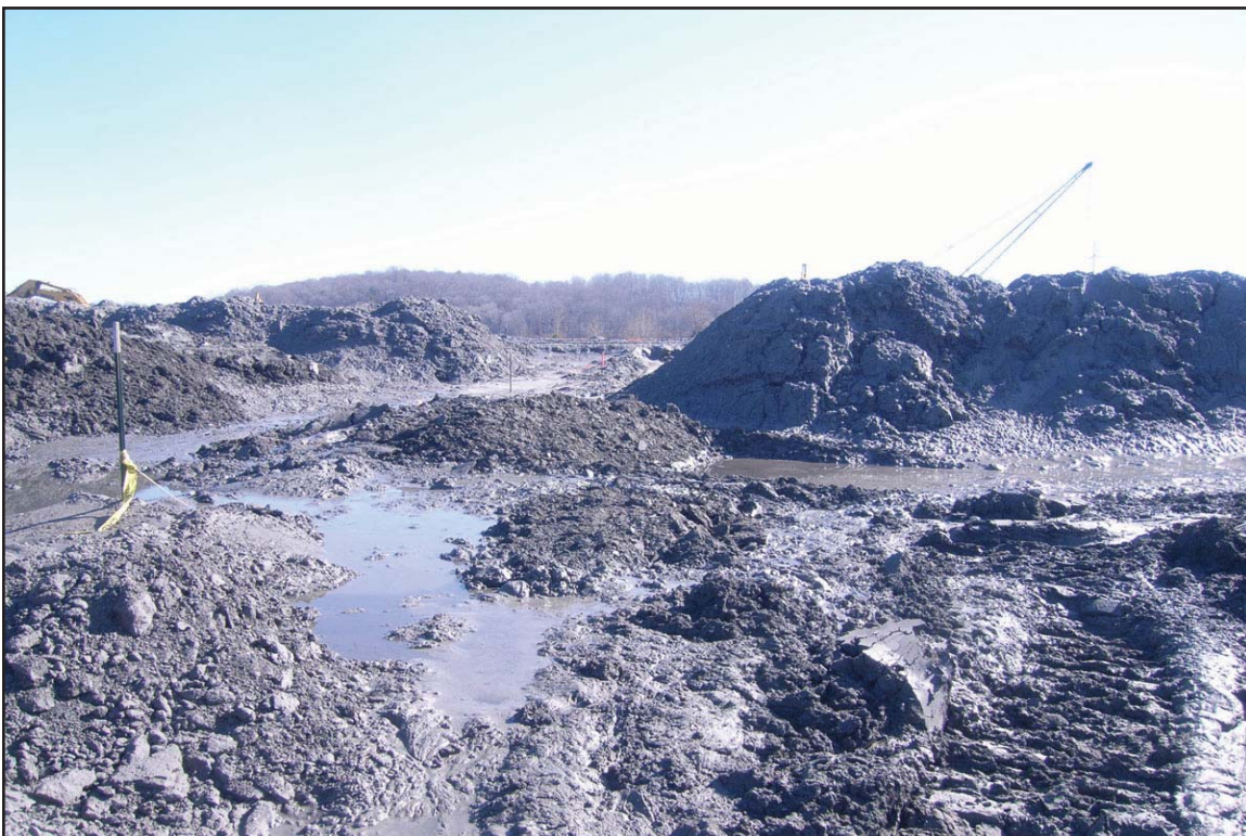
3J - Very wet conditions in Ball Field ash processing area during extended rainy weather. January 18, 2010.
