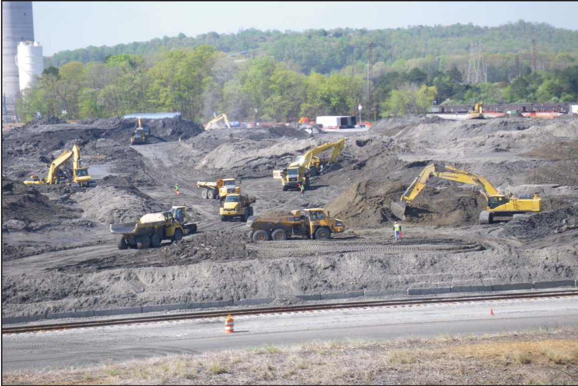
5A - Ball Field, temporary dry ash processing and storage of dredged materials prior to offsite shipment. April 12, 2009.
