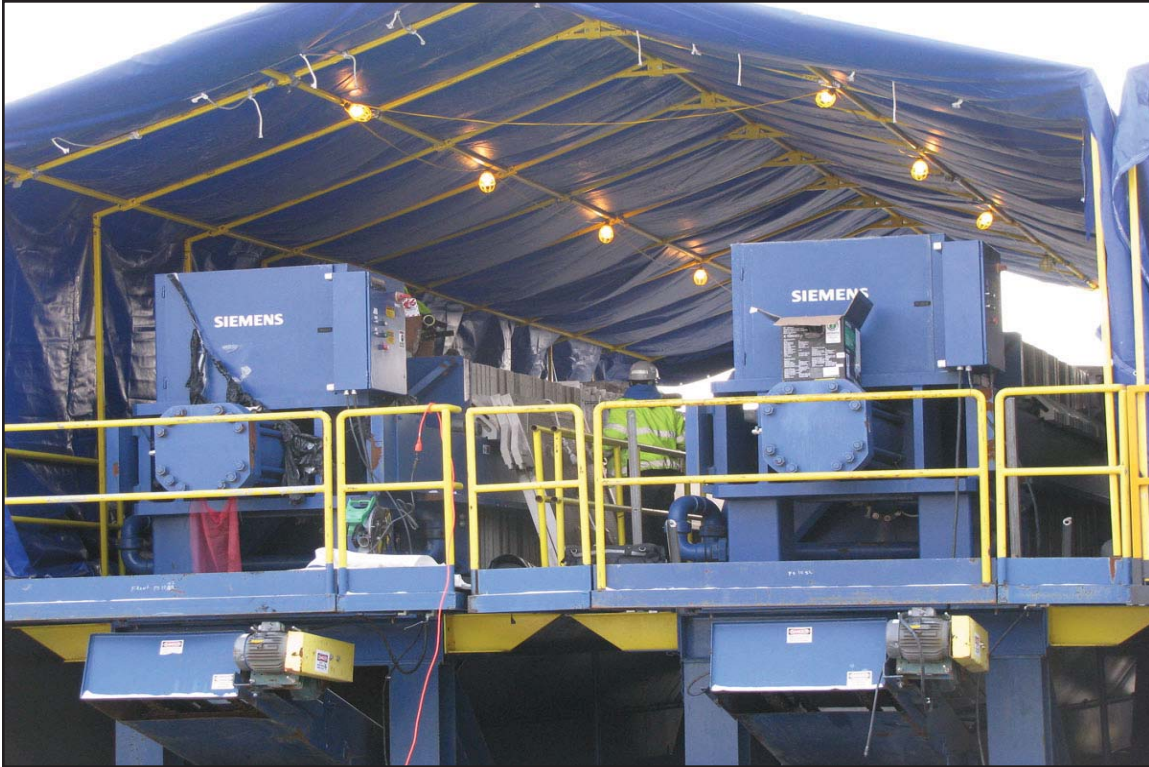
30 - Filter presses used for ash recovery from Ash Pond dredge discharge. January 9, 2010.
