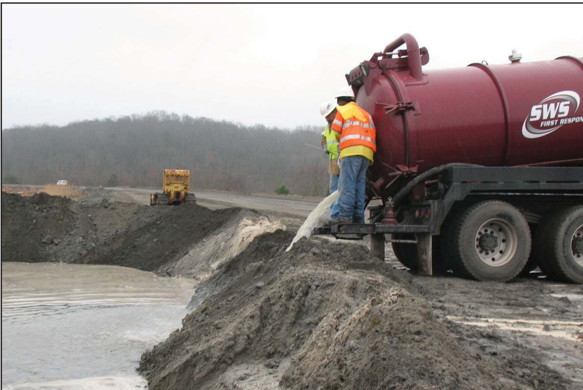
7L - Emptying vacuum truck into cenosphere pond (southeast corner of the Ash Pond). February 17, 2009
