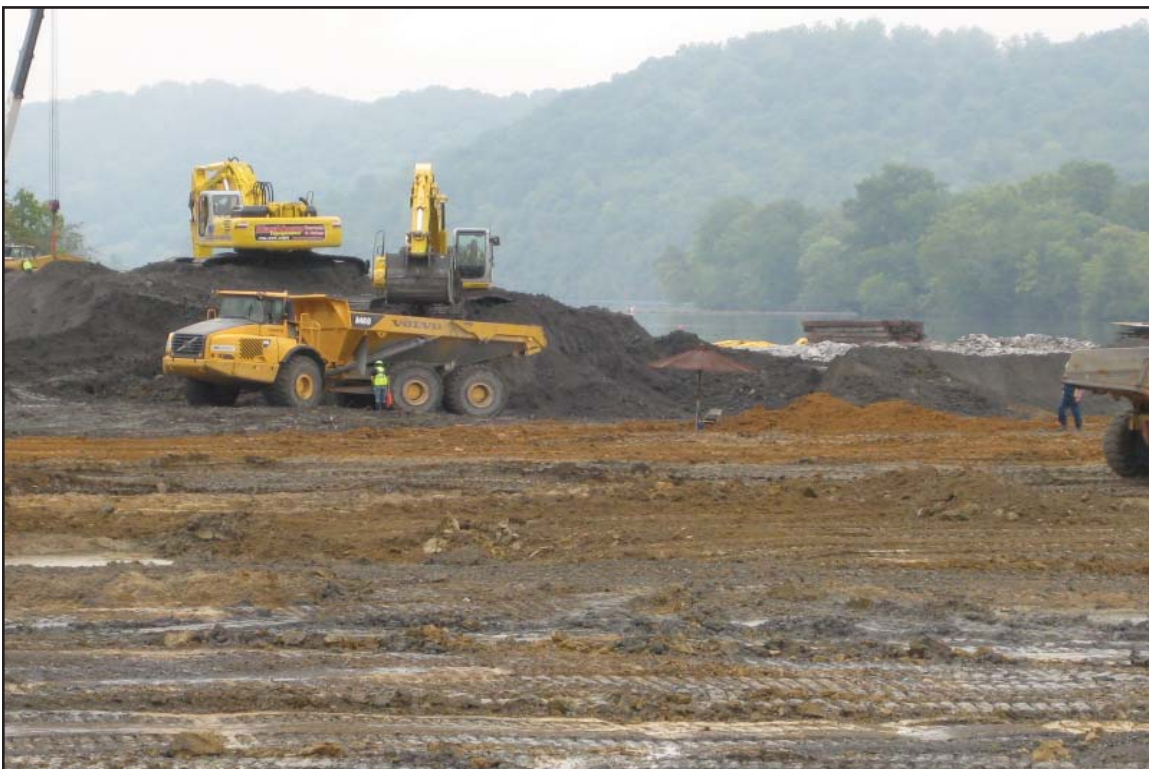
4D - Excavation east of Dike 2 using track-mounted backhoe excavators and rubber-tired articulated dump trucks. September 4, 2009.
