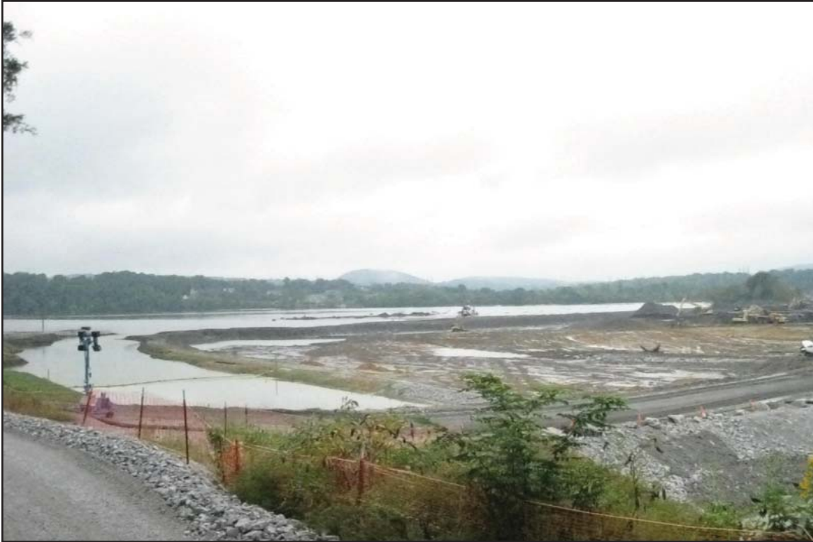
4I - Excavation east of Dike 2 nearing bottom of excavation (clean water ditch at left). October 18, 2009.
