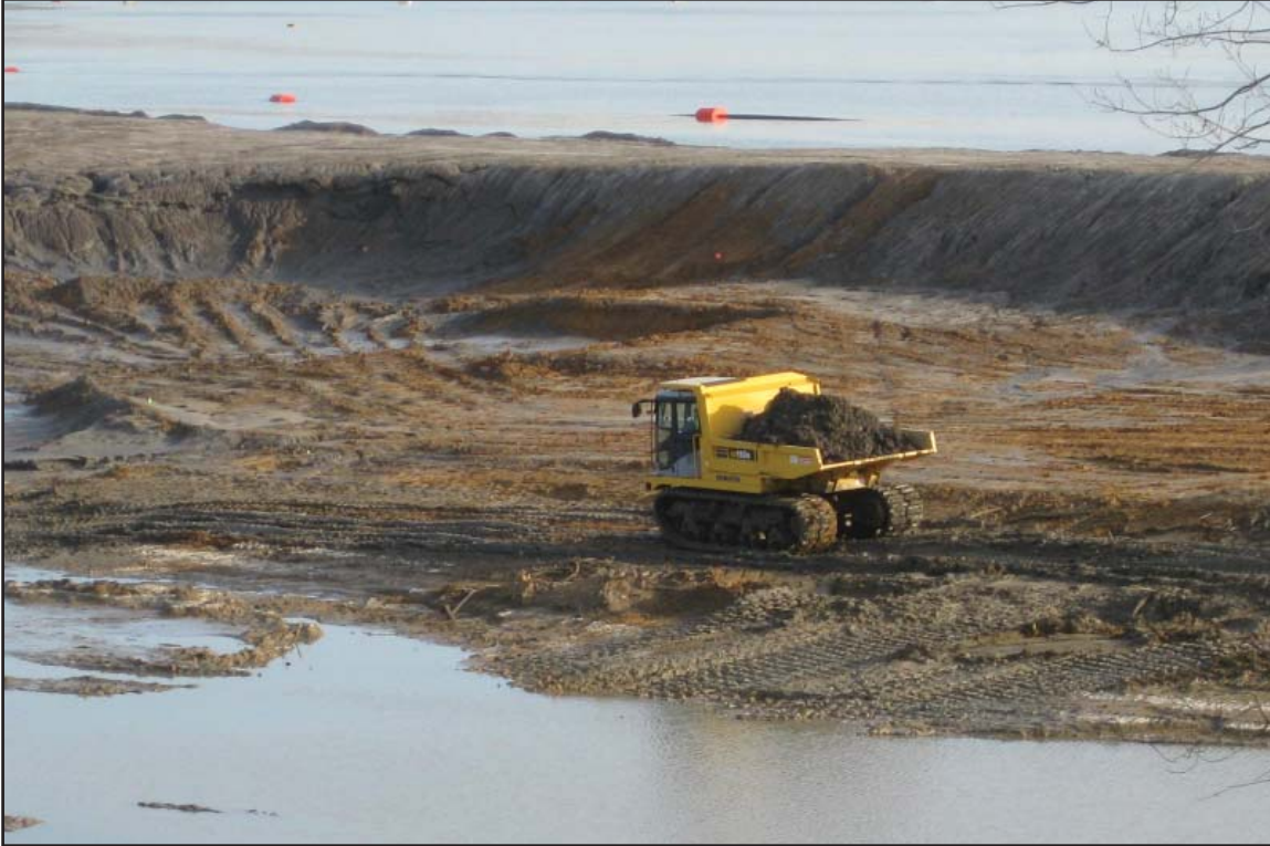
4G - Excavation east of Dike 2 using track-mounted light dump trucks in soft terrain. December 16, 2009.
