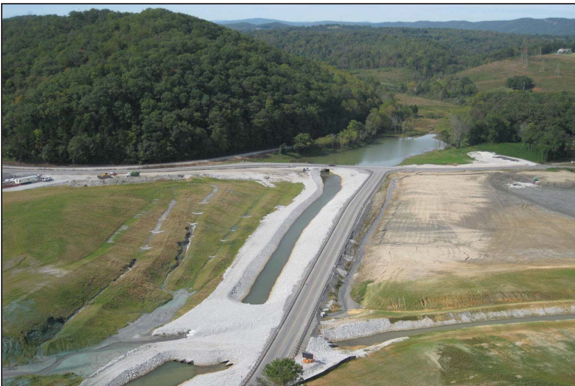
10B - Clean water ditch used to route clean stormwater around the ash in the Swan Pond Embayment. December 8, 2009.
