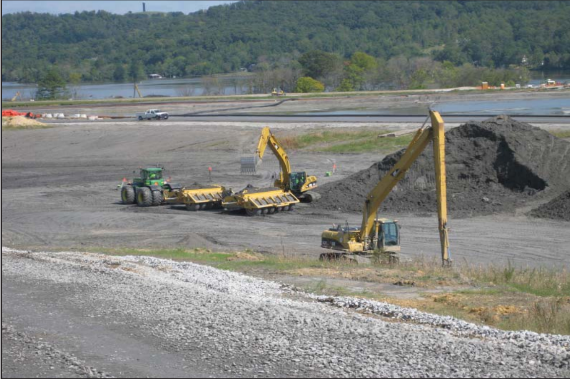
5G - Temporary storage of dry ash in “valley area” of Dredge Cell next to Dike D. September 30, 2009.
